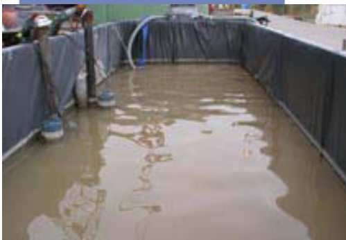
Water quality entering clarification system
