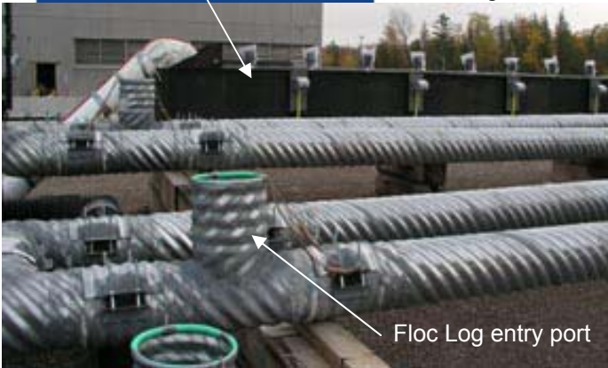
Pipe mixing system
