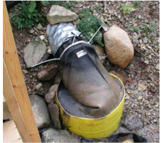
System exit point with filter bag Note dark water to left of bag ... indicating well-clarified water
