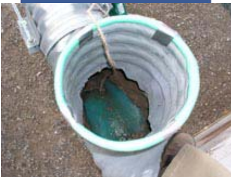
Polymer entry point with installed 706b Floc Log
